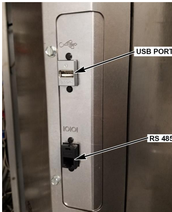
LOCATED ON BACK OF CONTROL DOOR
